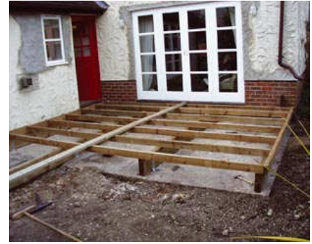
On this old concrete patio the deck frame is supported on 150 x 45mm (6" x 2") joists to lift it to the level of the French windows.
